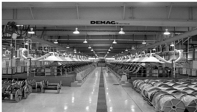
Fig. 11. Nickel foam production unit at the Inco Advanced Technology Materials, Dalian, China (Courtesy of V. Paserin).
